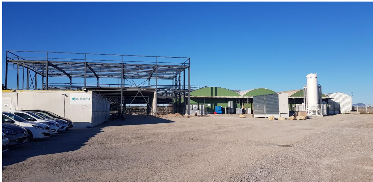
The world's first microalgae biorefinery under construction on Microphyt's site in Baillargues
